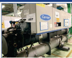
CHILLER SPRINGER CARRIER MOD. 30HXC
